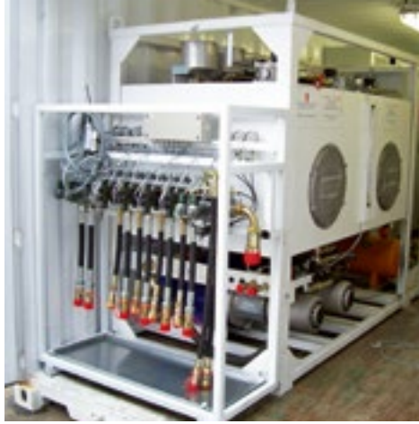
Hydraulikaggregat in Container
